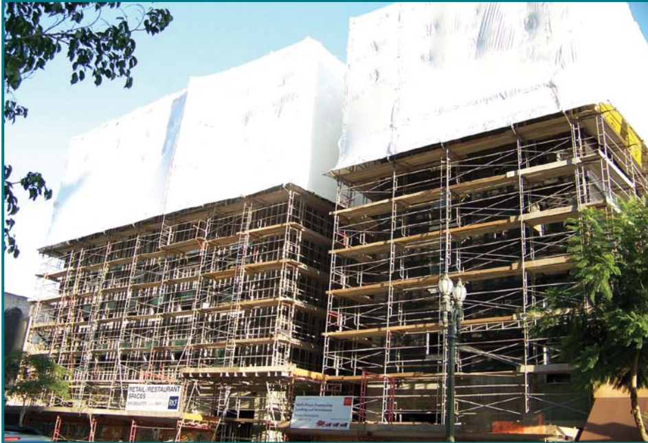
The Trust's New Genesis Apartments are currently under construction at 456 S. Main Street in downtown's Historic Core.
